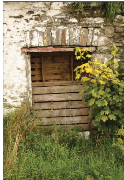
Plate 49 - Window opening west elevation B03
