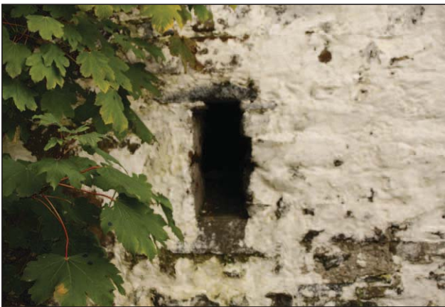
Plate 48 - Window opening west elevation B03
