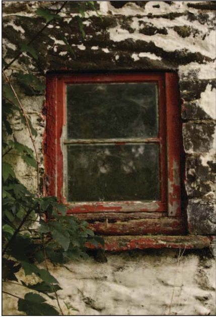
Plate 50 - Window opening west elevation B03
